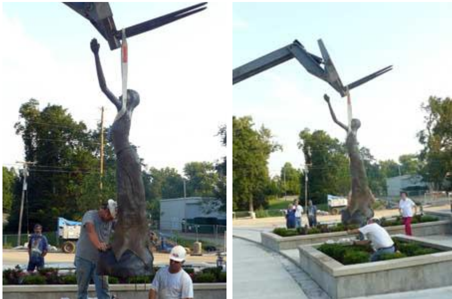
Construction workers place the St. Angela statue in to her new home.
